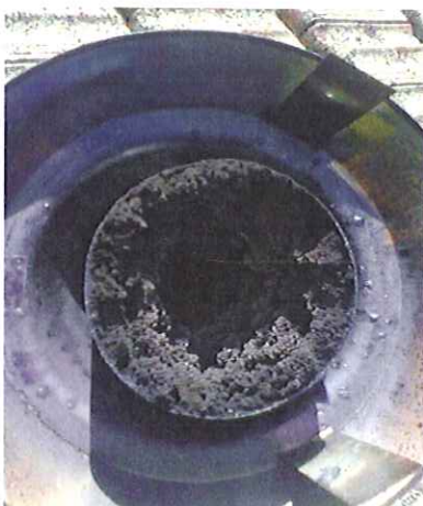
Creosote build-up in a flue (Australian Home Heating Association)
